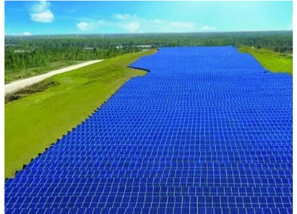
The Orlando Utility Commission's (OUC) Community Solar Plant on a site that includes a coal ash landfill.
