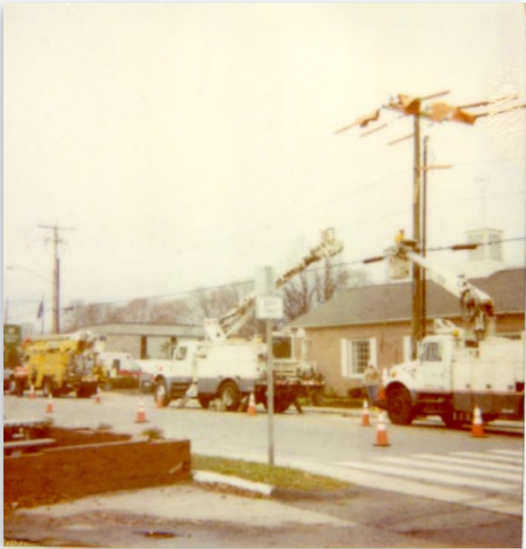
Spill from a Pole-Top Transformer
